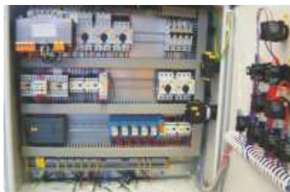
PLC controls / control cabinet
